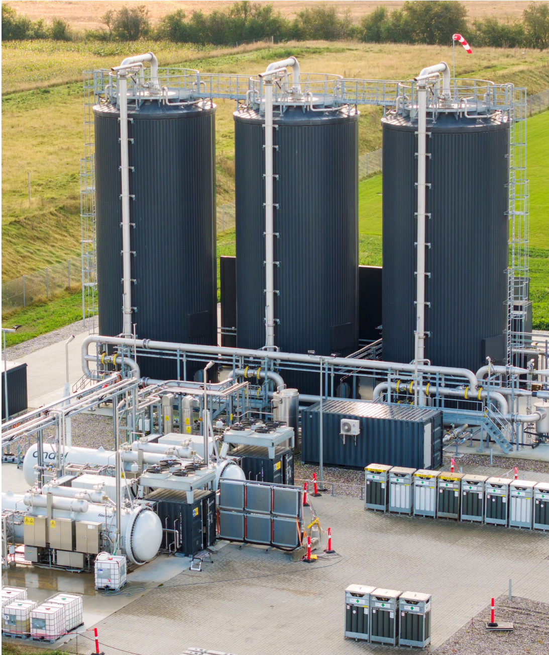
Andel and Nature Energy's joint Power-to-X plant in Glansager converts excess solar and wind power into hydrogen. The hydrogen, together with biogenic CO 2 , becomes e-methane, which is fed into the natural gas grid and displaces an equivalent amount of fossil natural gas.
